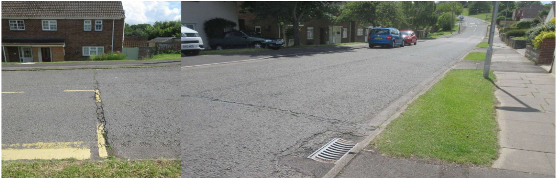
Trench opposite 32 Bishopdown Road. Further down the road a poor Drain Cover.
