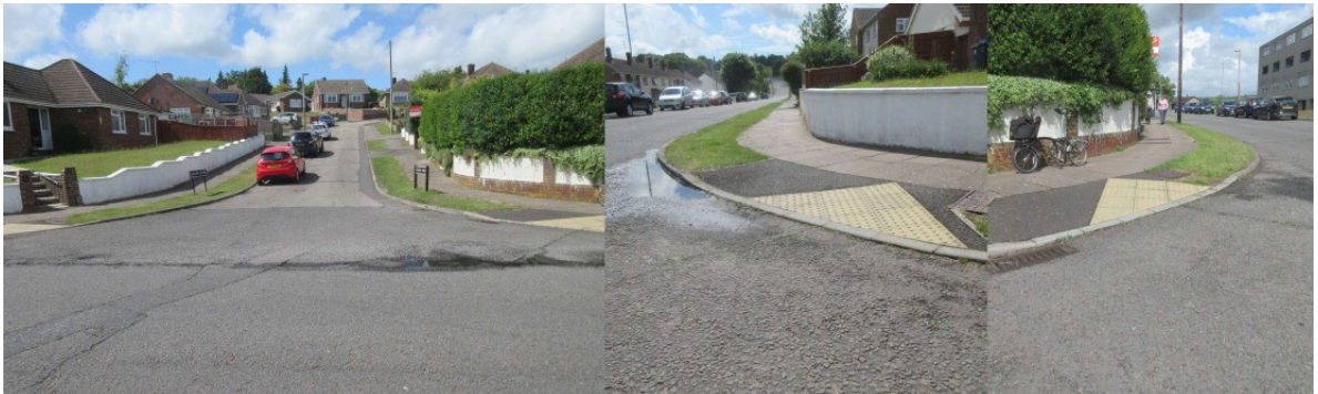
Entry of Bingham Road from Bishopdown Road. Poor road surface and drop kerbs not flush with road surface.
