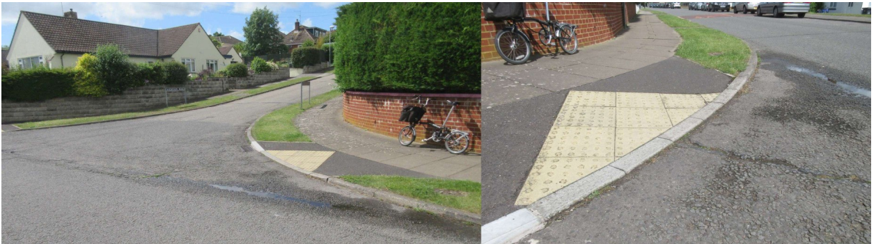
Footway crossing entrance from Bishopdown Road from Anderson Road. The road surface is poor, and the drop kerb is not flush with the road surface.
